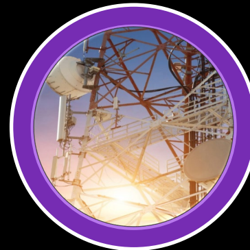
Communications Infrastructure and Datacenter
